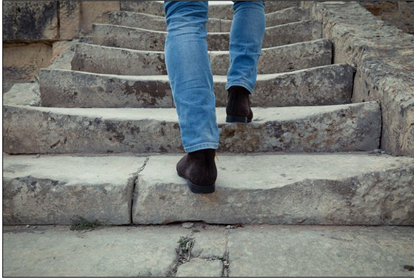
Figure 1: Example of steps that have uneven wear after long term use.
